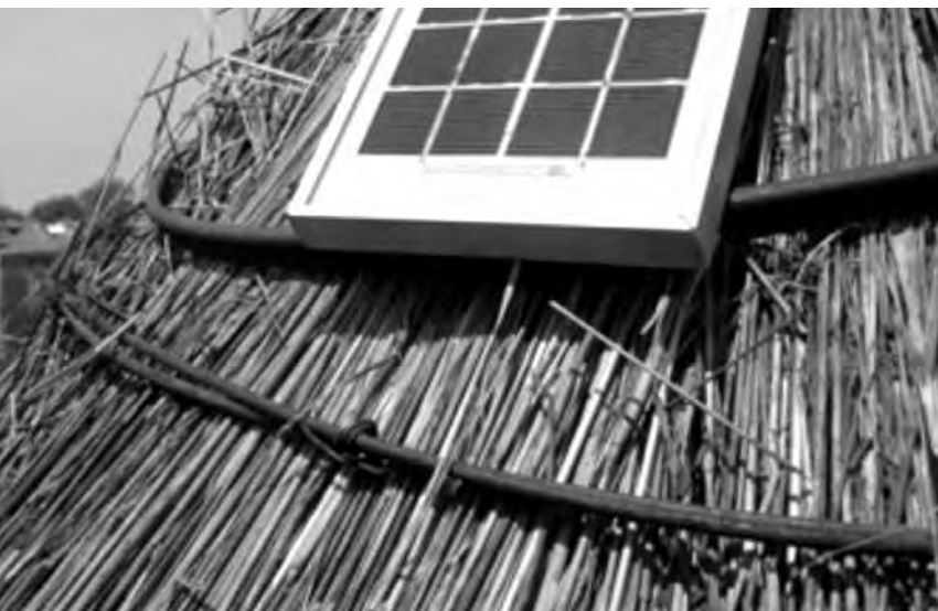
Off-grid solar system. 24
