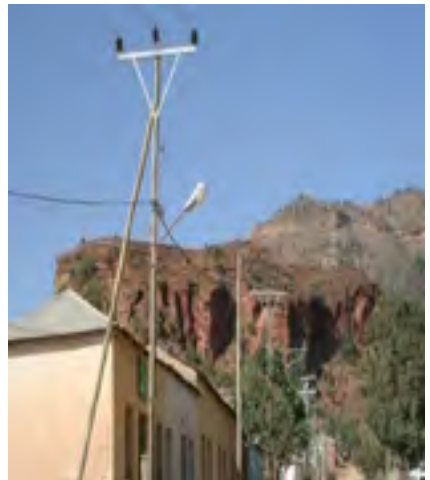
Figure 2: Extension of power lines in rural areas of Ethiopia
